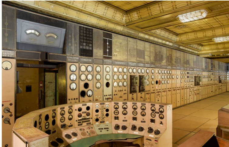
Figure 2. A control room from the 1950's.
