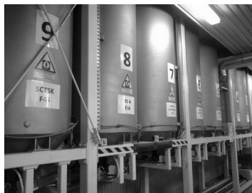
Figure 7: Silos and automatic storage compound system
