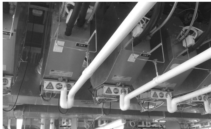
Figure 3. Individual ATMs for each TIEQ cubicle workstation.
