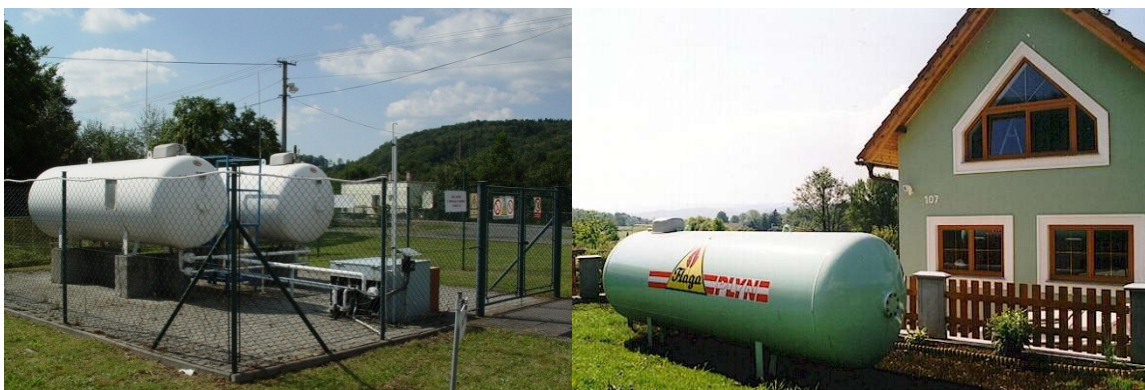
Figure 1: LPG filling station in a plant and that for domestic use
