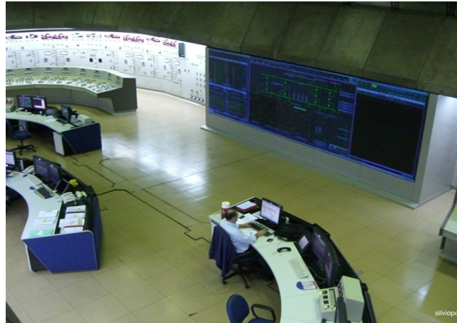
Figure 1 - Room of Electric Power Operation and Control Center
