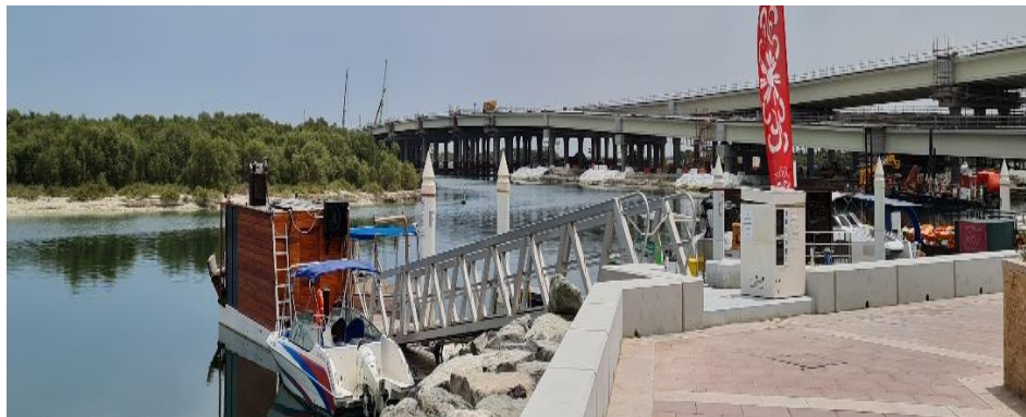
Figure 1. Construction of the new bridge crossing the Eastern Mangroves to Umm Lafina and Al-Jubail Islands.
