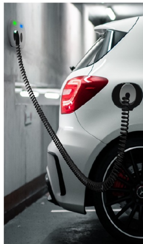
Figure 5: Portable level 2 charger with coiled cable: The second version.
