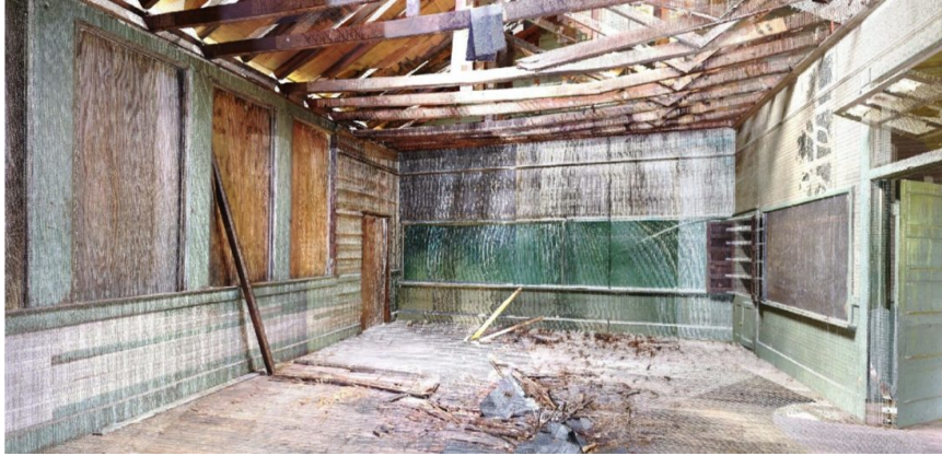
Figure 1: LiDAR image of Tankersley school revealing construction details and extent of decay (image provided by author).
