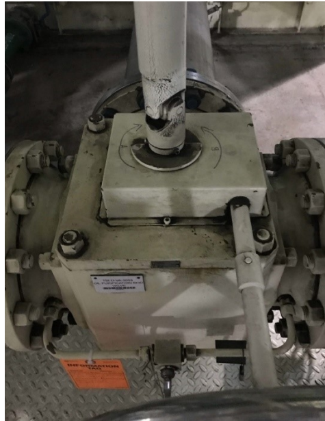
Figure 1: 6-way valve (Public Service of Colorado).
