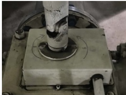
Figure 2: Closeup of labelling on the valve (Public Service of Colorado).
