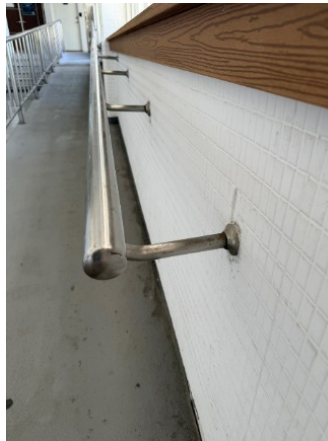
Figure 4: Current state of the ramp handrails.
